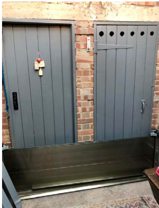
Photo: flood barrier covering two doors, Swithland
