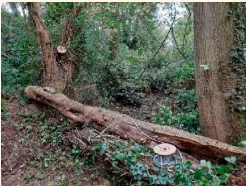
Photo: Leaky dam upstream of Breedon
